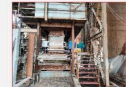
Relocation of AF Equipment's
